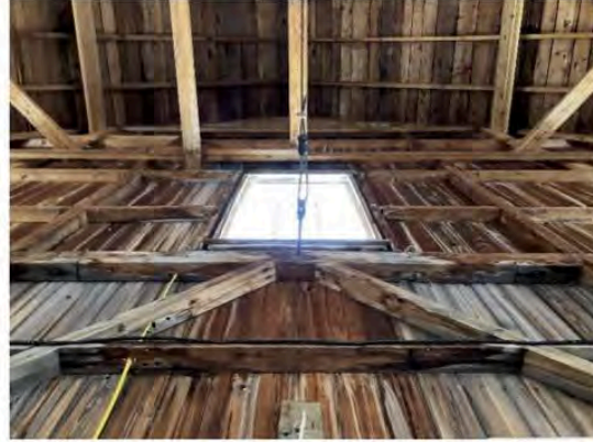
8) Interior – A cable was previously installed to tie the east and west end walls together; walls are out of plumb differing amounts
