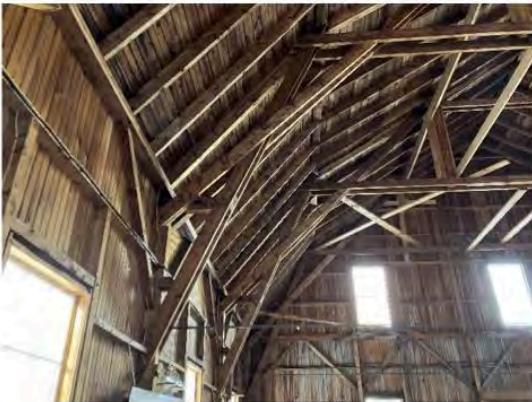
11) Interior – Truss performance relies heavy on connections and bracing; failures were not observed although the assembly appears light
