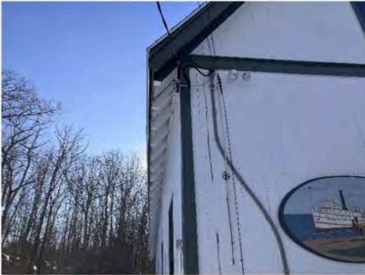
13) Exterior – Wall at eave is not linear; walls pull in at trusses and bow out between, suggesting deficiencies
