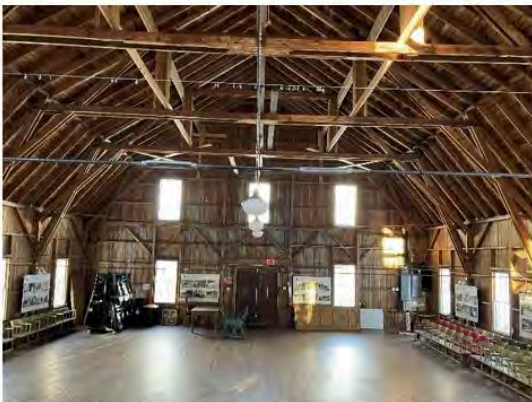
5) Interior – Assembly hall with stick-built gambrel trusses and steel tie rods; view looking east toward Shore Road
