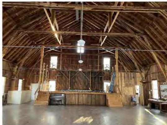
6) Interior – Assembly hall with stick-built gambrel trusses and steel tie rods; view looking west toward the stage
