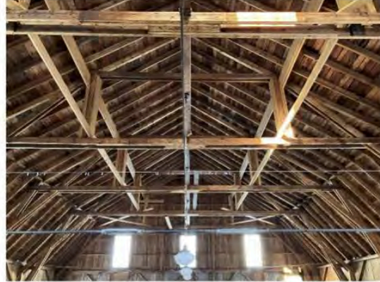
10) Interior – Typical clear-spanning trusses were previously reinforced with additional vertical and horizontal members
