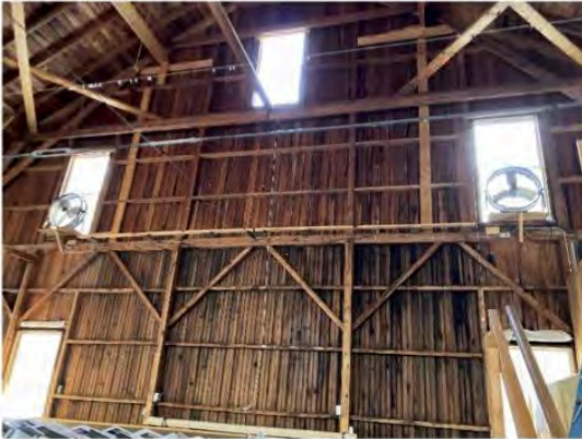
7) Interior – Gable end walls are lightly framed; walls are out of plumb; wall bracing is likely deficient
