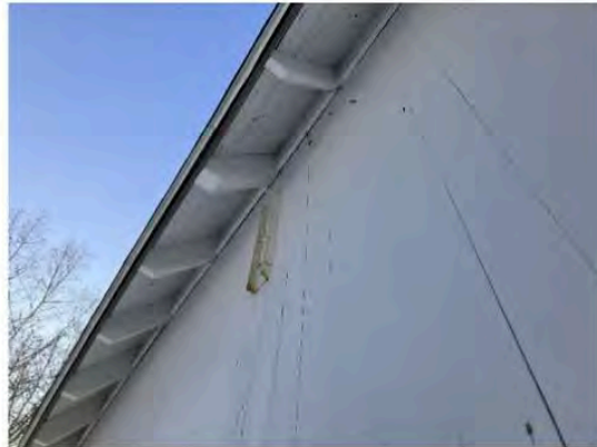
14) Exterior – West truss has a raised steel tie-rod with a steel bearing plate on the exterior; changing the rod elevation impacts the structure
