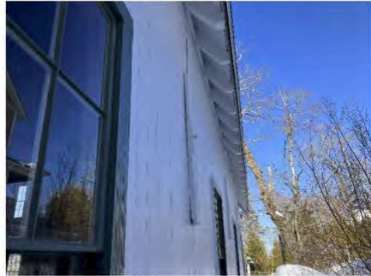
12) Exterior – Steel tie-rods extend to the exterior of the building and attach to wood or steel bearing plates; wood plates are bowed
